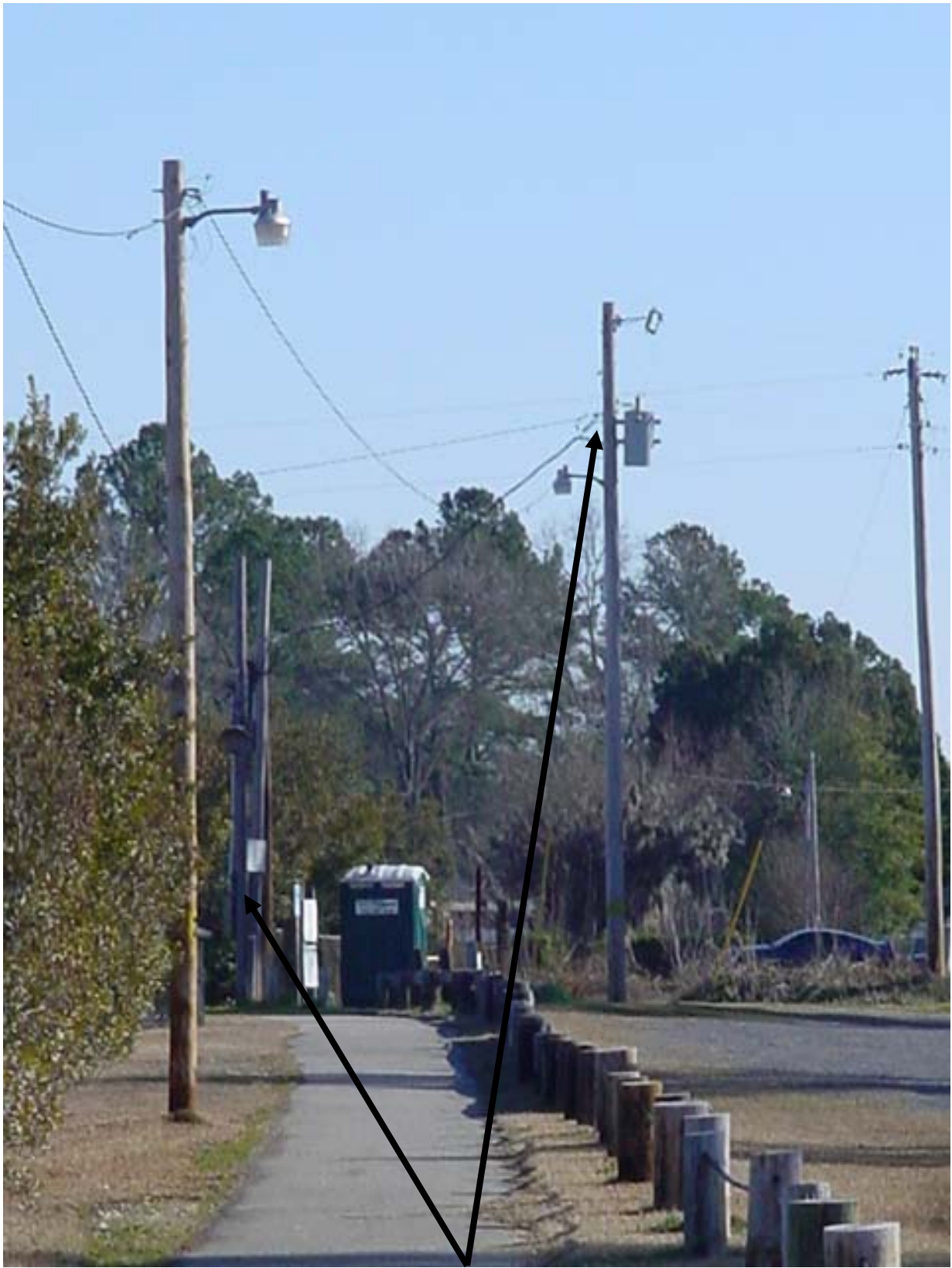
EXISTING ELECTRIC SERVICE ENTRANCE
